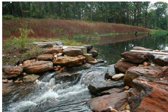
Figure 6. Concrete weir constructed at the top of the channel reach adjacent to Ritchie Hwy and upstream headwater wetland.
