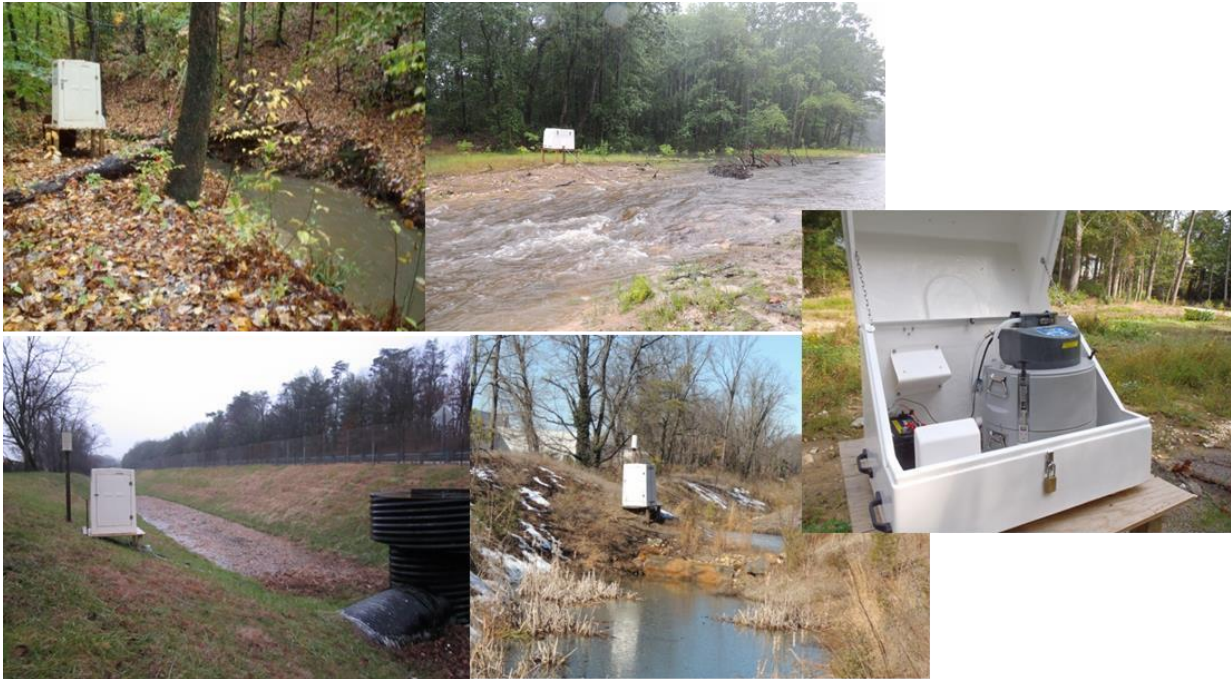
Figure 16. Automated water sampler in a protective housing at Cypress Creek before restoration (top left) and after restoration (top right). Sampler installed at the Leelyn Dr. stormwater structure before retrofit (bottom left) and after it (bottom right). The sampler type used, ISCO 6712, is shown on the far right photo.
