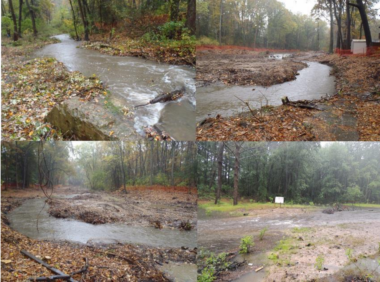
Figure 5. North Cypress Creek channel before restoration implementation (top left), during the riparian forest removal (top right, bottom left, and at the end of construction in the following spring (bottom right).
