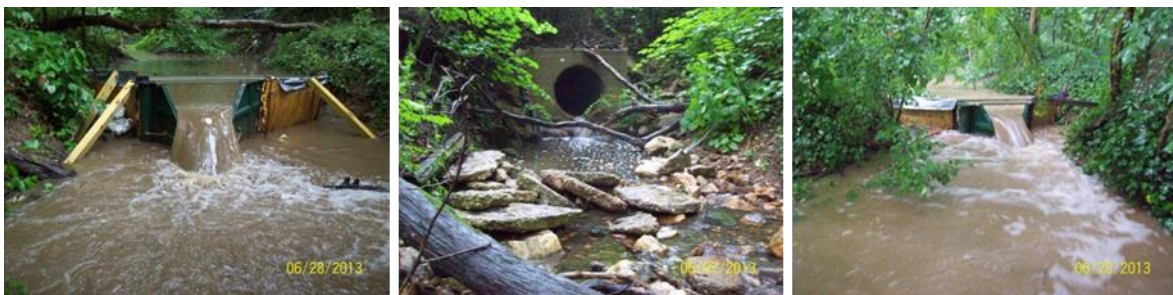
Figures (photos) 2a, b, c. From left to right: RSC catchment flume, RSC catchment culvert, and control catchment flume sampling stations in the pre-construction period.
